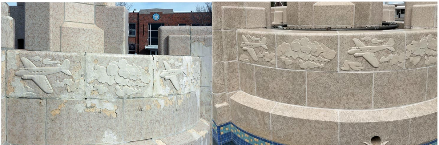
Figure 4 - Airport Fountain details, before and after restoration (Left image courtesy of Retro 106.5 website , right image courtesy of author)
